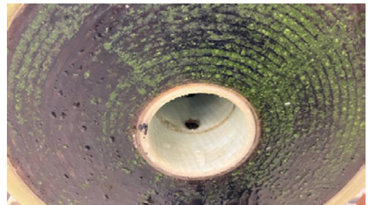
Fouling of membranes
