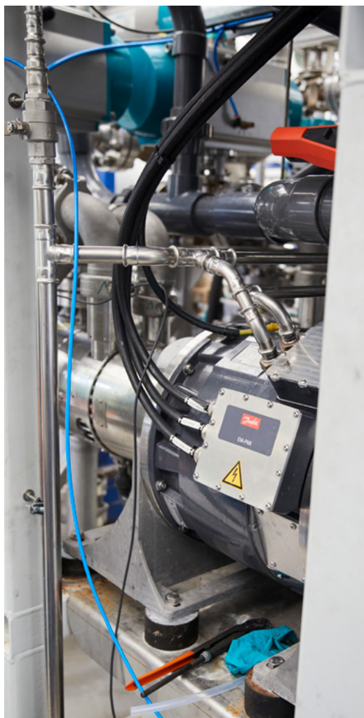
Turbine Pump Unit
